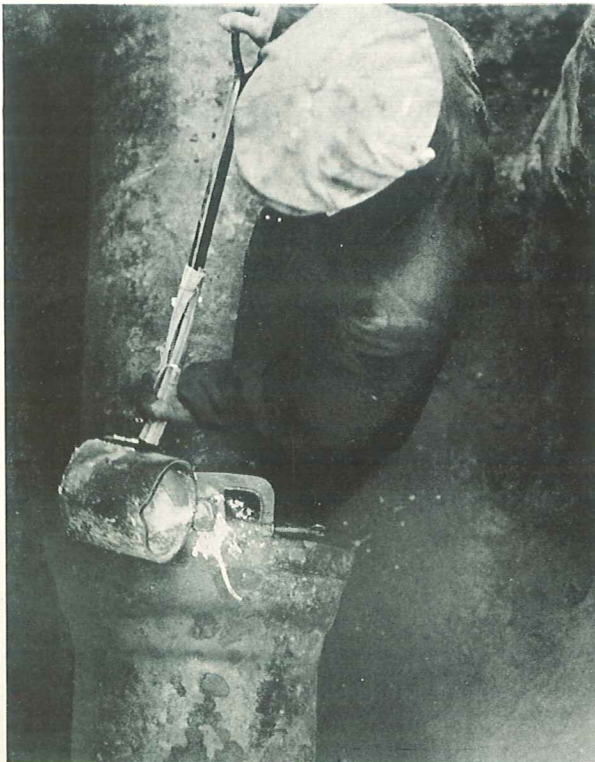
Workman pouring molten caulking lead into a joint in a cast iron water main.
